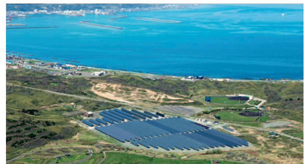
Wakkanai Mega Solar Power Station (Wakkanai)
